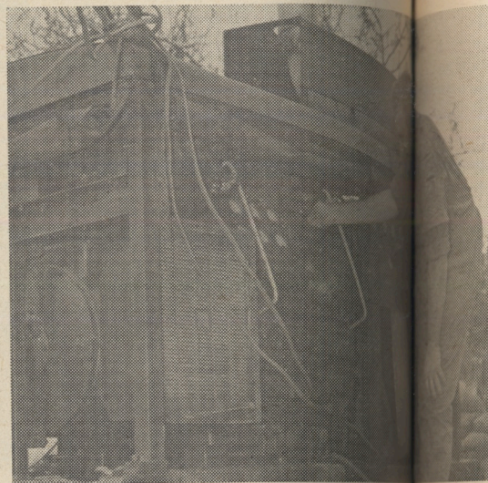
The man with a flair for 'big engines' Stephen Mooney from Lisdonvarna, Co Clare is doing a maintenance check on the generator. While Stephen remains at his post the men from B Coy need have little worries about a power failure as the eye of the master will quickly detect any fault.
